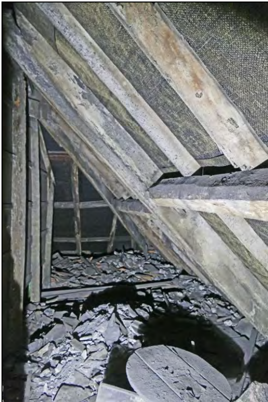
Illus. 21: North roof slope of the attic of the Northern Building, looking west towards the hipped corner; note the roughly-chamfered staggered butt purlins. This is a less-altered section of roof and may be of relatively early post-medieval date.
