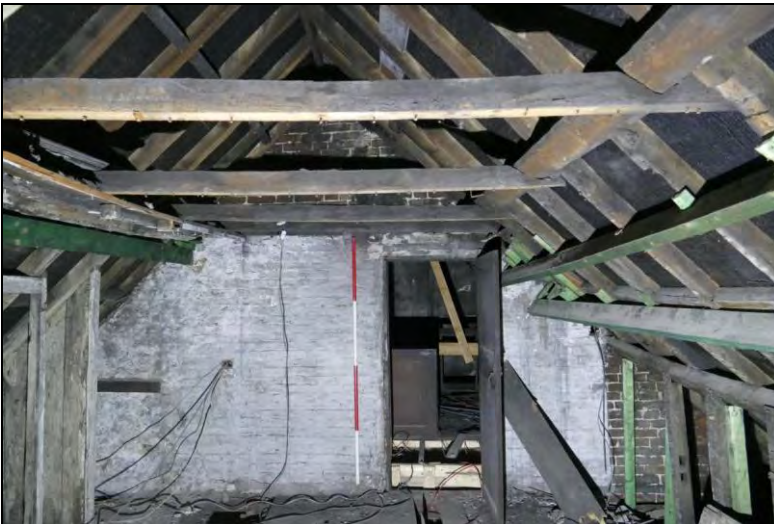
Illus. 19: Attic of the Southern Building looking north, showing the old two-panel door into the attic of the Northern Building, and the collars with notches to carry purlins; these are probably secondary (see the cuts for earlier purlins on the rafter).
