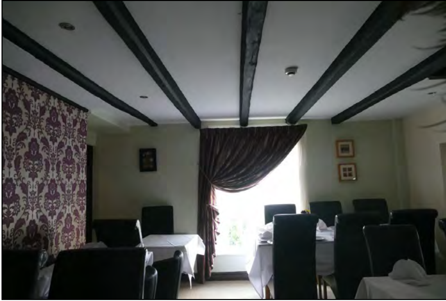
Illus. 17: Southern Building at first floor level looking west, showing old ceiling beams
