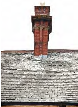
Figure 4.44: Lake District slate on the roof of the old Gas Board building
