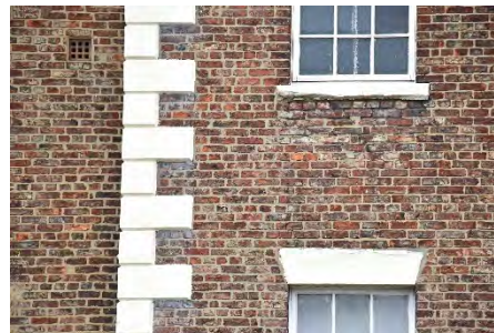
Figure 4.39: Hand cut bricks in the facade of the Northern Centre for Photography
