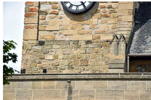
Figure 4.14: Differential weathering on stonework in the Minster
