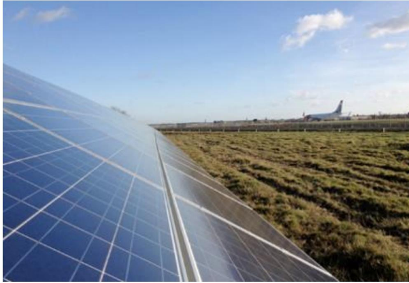
Figure 2: Solar Array next to Gatwick Runway (Business Green, 2013 8 )
